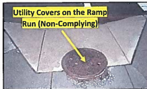
Figure 39: Non-Complying Utility Covers
