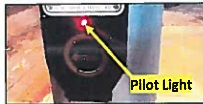
Figure 77: Pedestrian Pushbuttons with Pilot Light
