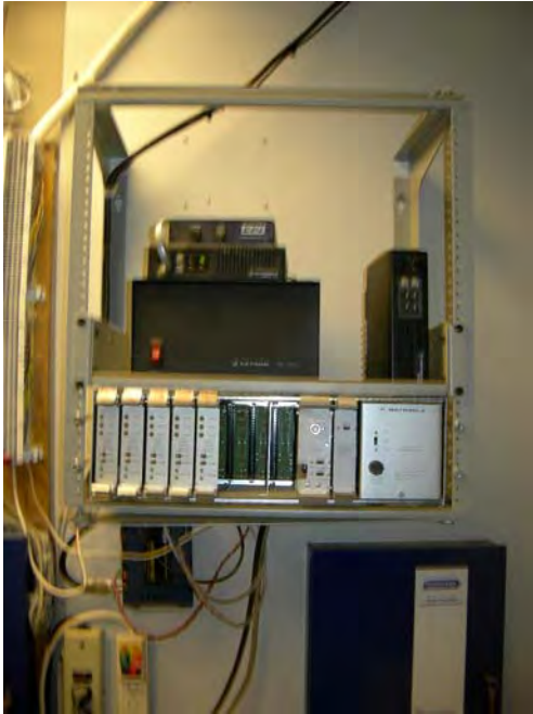
Existing setup on the rack
