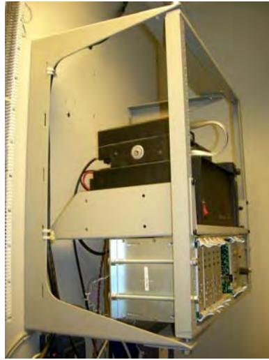
Side view of rack system in closet
