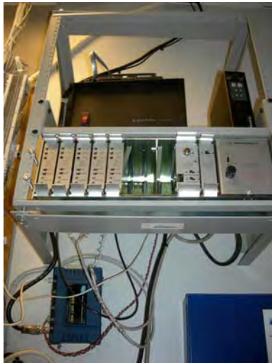
Under view of rack system in closet
