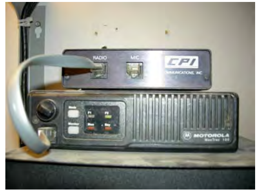
Existing CPI tone remote chassis and non compliant MaxTrac 100 radio
