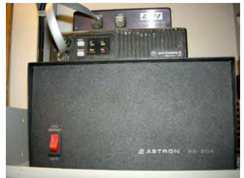
Existing CPI tone remote adapter chassis, mobile radio that needs to be replaced and Astron RS-20A power supply
