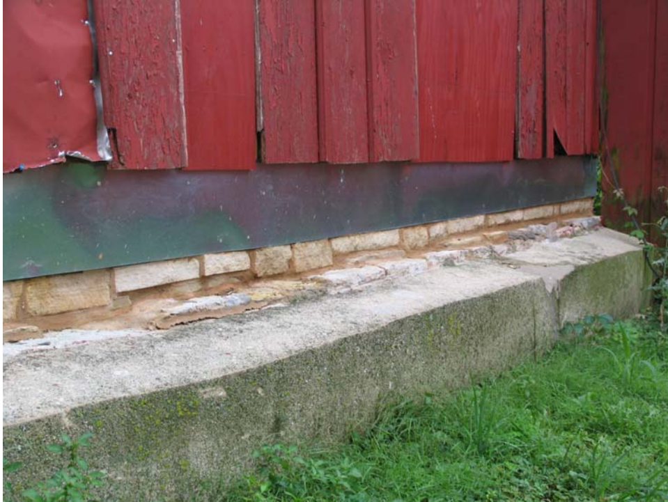
Close-up of modern stone used to level the foundation, over original poured concrete foundation.
