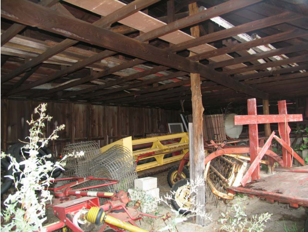
View to northwest. Interior of cattle shed attached to south end of barn.
